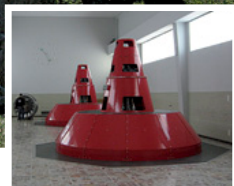
▲ Machine hall at HPP Gordola
