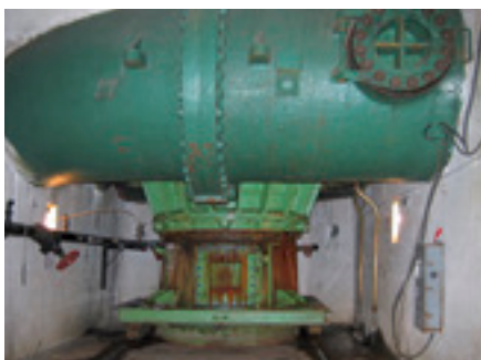
▼ Draft-tube cone and lower cover before refurbishment
