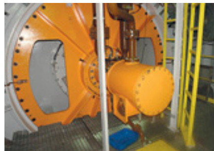
▲ Bulb generator at HPP Santo Antônio
