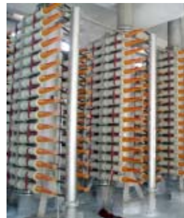
Andritz TC-133 cleaner plant.
