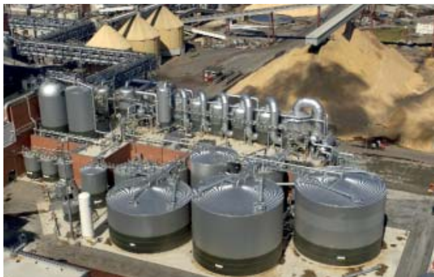
The most advanced evaporator plant in the world is operating at Pietarsaari. Supplied by Andritz, the plant evaporates 1050 t/h of water and produces firing liquor at 85% dry solids using a Liquor Heat Treatment Concentrator.
