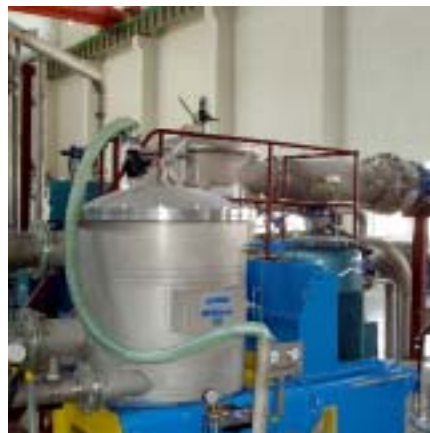
Thick stock screening system (0.15 mm slotted baskets) at Yanzhou.
