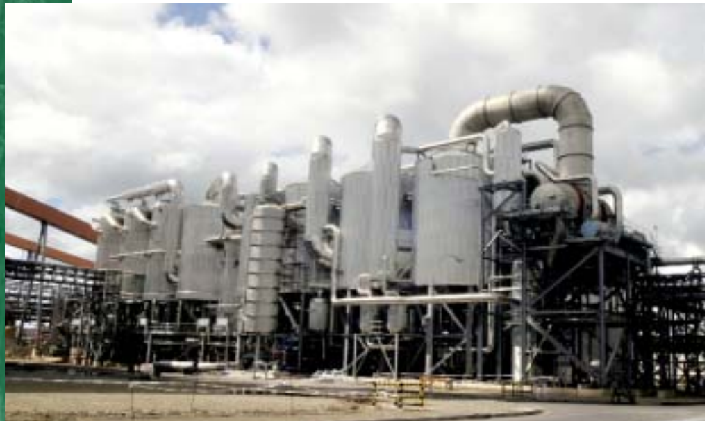
The Andritz evaporation plant at Valdivia removes 876 t/h of water and delivers 78% dry solids black liquor to the recovery boiler.
