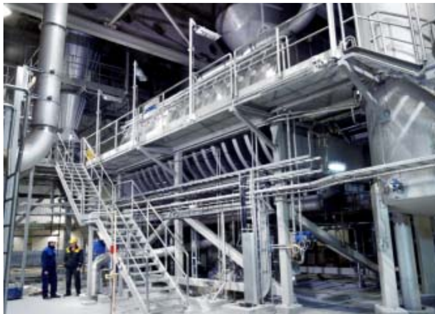
The white liquor plant supplied by Andritz is the world's largest at 10,000 m 3 /d of white liquor production. Lime mud for the kiln is separated, washed, and dewatered in a special disc filter, the Andritz LMD-Filter™ (above), which is new Andritz technology. Markku Lankinen (left) of Andritz and Kaj Nordbäck, Power and Recovery Plant Manager at Pietarsaari stand in front of the new filter.
