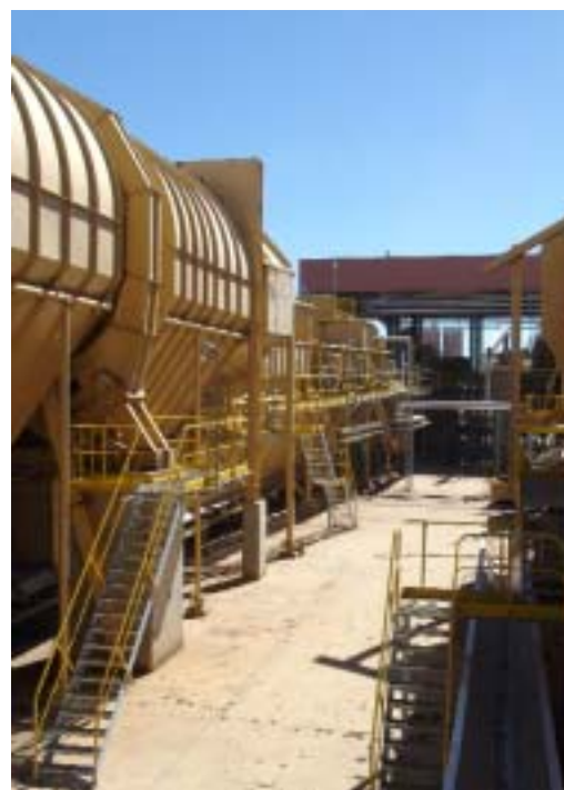
One of the debarking drums on the new lines at Valdivia. Each drum is 5.5 m in diameter and 35 m long.
