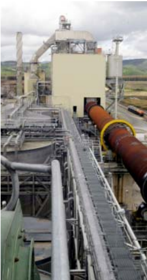
The Andritz 7600 m 3 /d white liquor plant for Valdivia started up on schedule and exceeded nominal production within two weeks of start-up.
