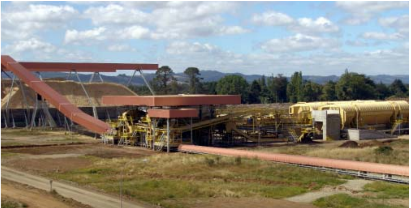
The Andritz two-line debarking and chipping plant for the greenfield Valdivia mill. Andritz's scope also included chip storage and reclaiming.
