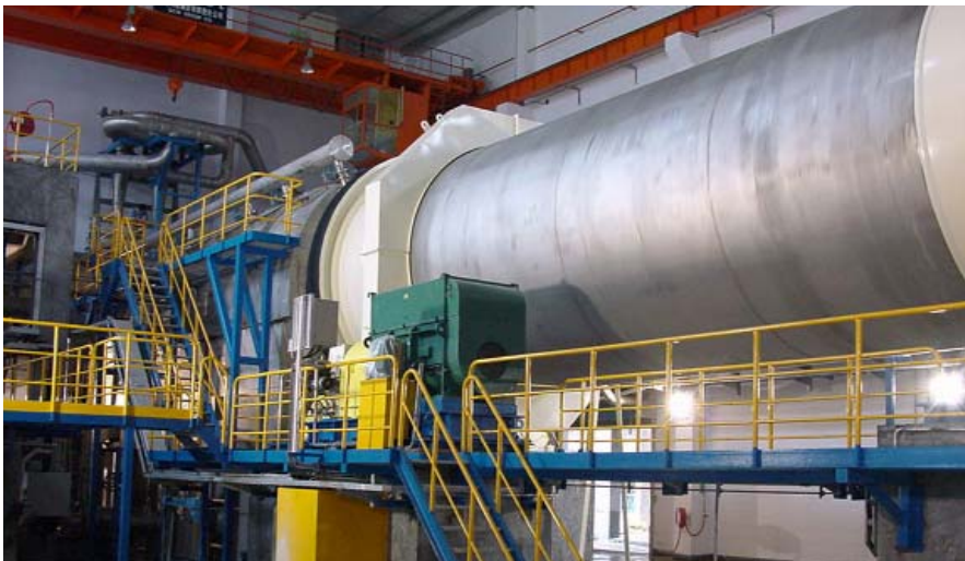
The new FibreFlow® Drum pulper at Nanping has a capacity of 320 t/d.
