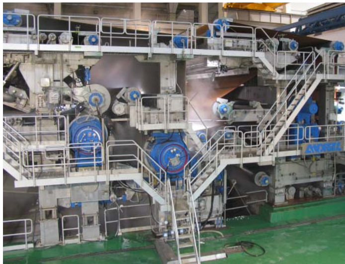
The pulp machine has Andritz's advanced twin-wire forming technology. Dewatering in the press section is accomplished by a three-roll Combi-Press, followed by a double-felted shoe press.
